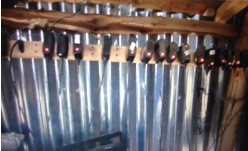
Figure 3.8. Mobile phones being recharged at the charging unit providing service to Amayo and surrounding kebeles .
